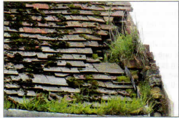
The state of part of Abbey Mill roof in 2013
