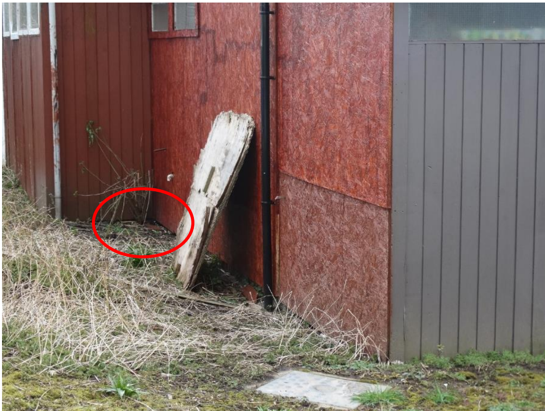
Or appear to have little or no foundations at all (Youth Hall East side).
